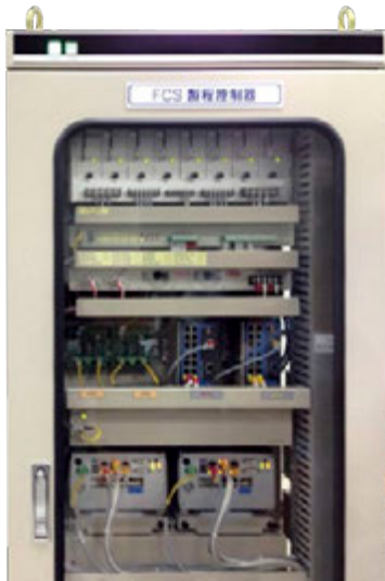
Figure 1. NEXCOM NISE 3660 is installed in the cabinet as a DCS controller.
